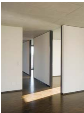
Finished edges on partition walls help avoid damage to edges and appear more moveable.
