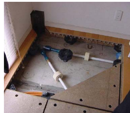
Using a raise floor system allows electric and utilities to be easily rerouted upon renovation/change of tenants.
